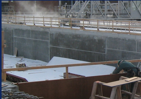
Waste water treatment plant, Canada
