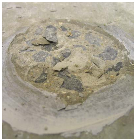
Fig. 6b Concrete surface after a pull-off test
