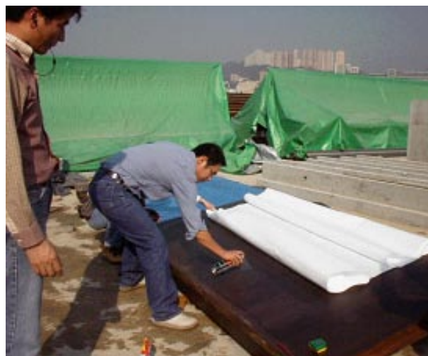
Figure 9. Test formwork is prepared with the competing product on the left and Formtex ® on the right.
