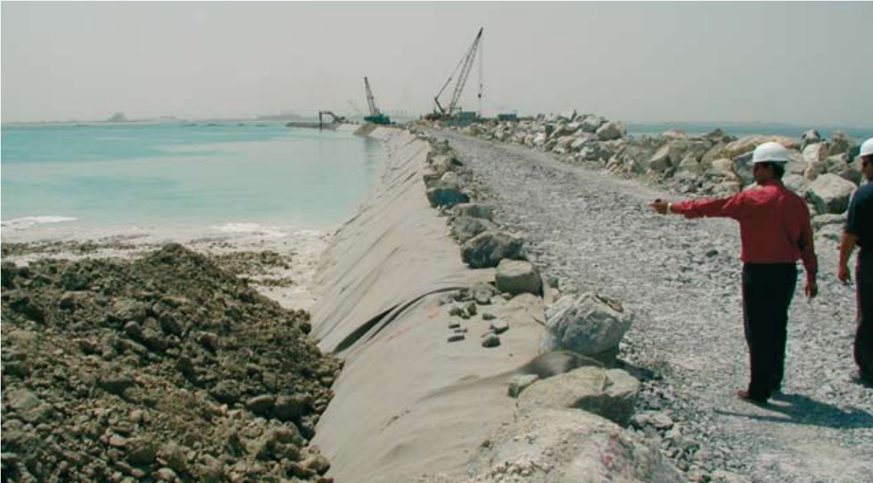
Source: Palm Island, Dubai. Installation of Fibertex F-650M. The Fibertex Geotextile will be covered completely with gravel and sand.
